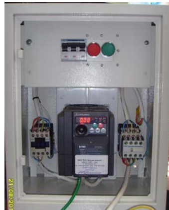
Fig. 8. Frequency converter Mitsubishi FR-D740 for traffic control scraper conveyor.
