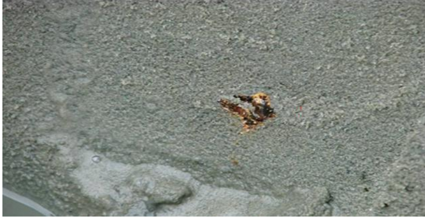
Pic. 1. Photo of the condition of damaged lands
